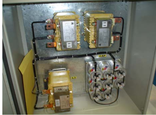
Photo: 20HP single phase low pass harmonic filter
